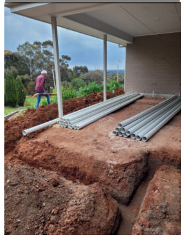
Roger's Just Finished Digging All Those Trenches, Now Heading Out The Front For More (At Least That's What It Looks Like)
